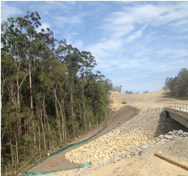
Fig. 1-4. Construction of highways through natural areas involves clearing and reshaping the landscape. Photo: Author/Sandpiper Ecological.
