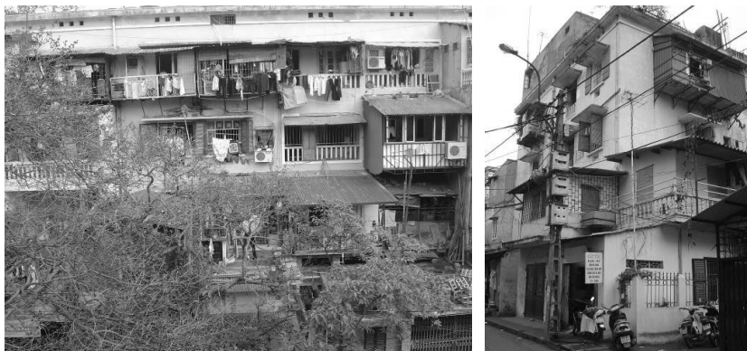
Fig. 1-2. Chuong cop or “tiger cages”—additional structures that have broken the concrete walls of the KTT. 11
