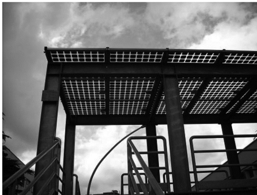
Figure 1: View of the PV array
